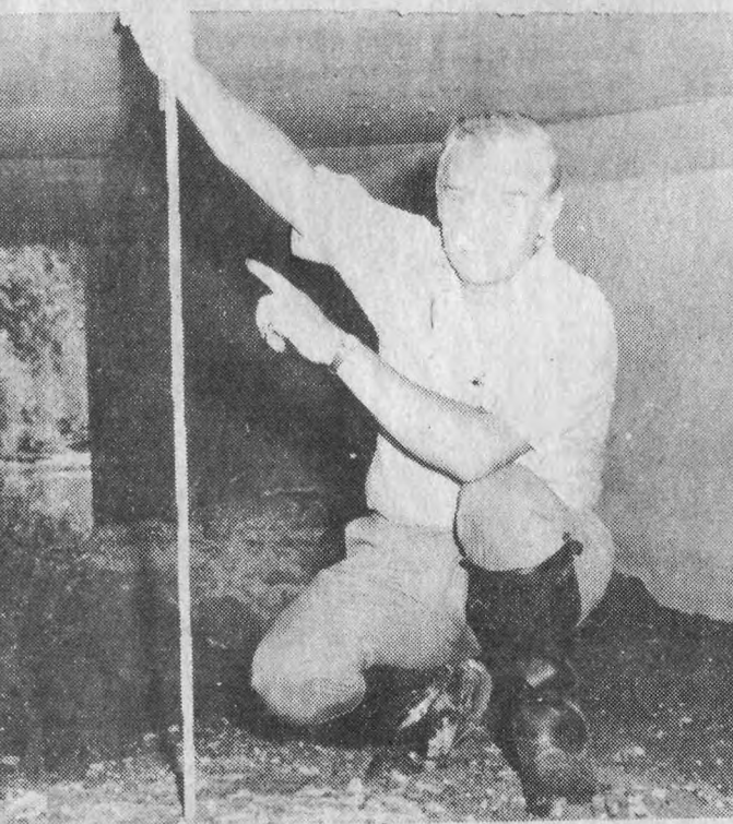
SILTED DIMENSIONS ... Public Works and Engineering Director John F. Allaire, Jr. shows how silt has stopped the water flow on Pumpkin Patch Brook. The bed should be 10 feet below the ceiling of the bridge, but muck and gravel have reduced the level to four feet.
