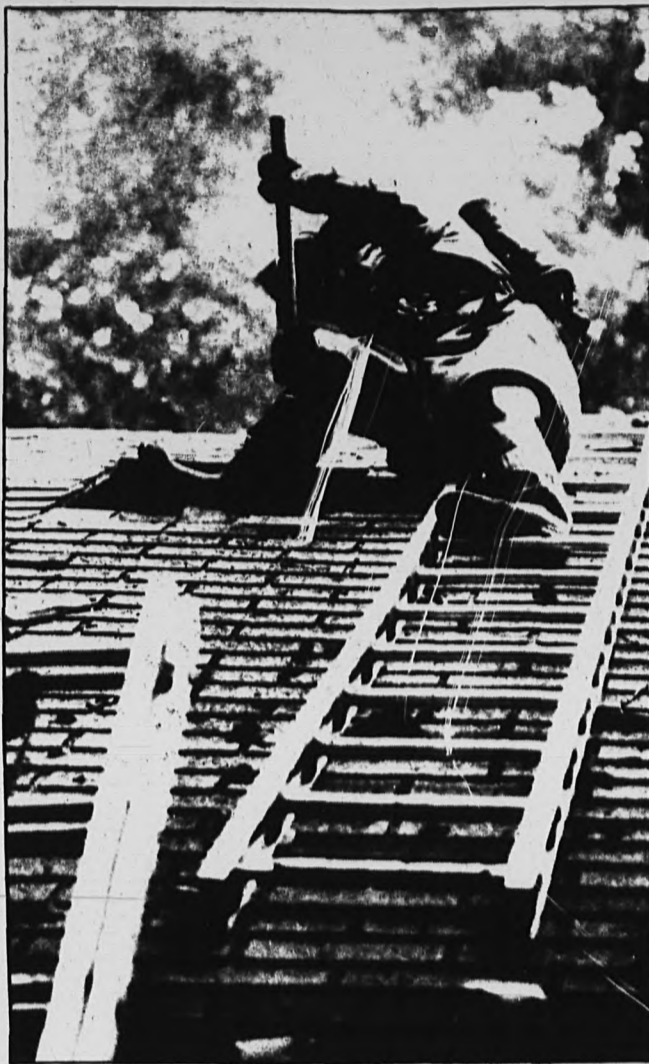
HOT WORK — An unidentified Lincroft fireman pokes through a hole chopped in the roof of a West Front Street home in Middletown to help put out a fire that gutted most of the interior. No one was injured, but one of the owner's dogs perished in the blaze.
