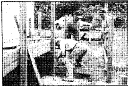
Volunteers work on the handicap ramp for Burnap Cottage as part of the restoration project.
