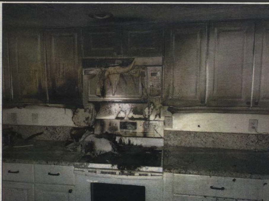
A fire on March 22 in the Sandalfort Beachfront Condominium resulted in 80,000 in damages.
