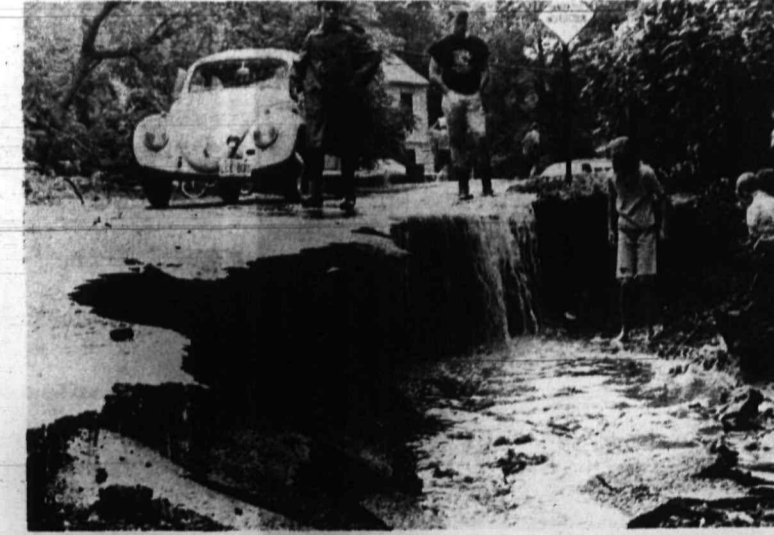
END OF THE ROAD - A road at Clearwater Swim Club near the intersection of Division avenue and Blackburn road crumbled under the pressure of the heavy rains Monday morning. Such sights were common about the city following the rain. (Rennie Coit Photo)
