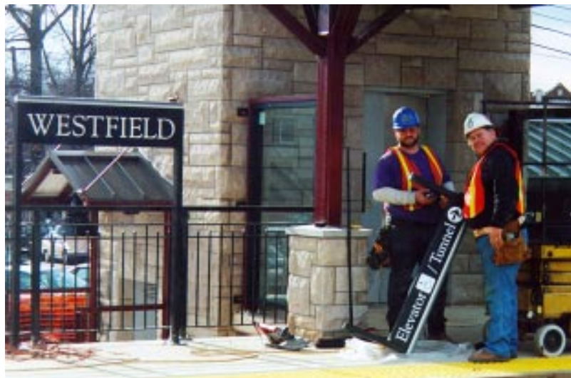
David B. Corbin for The Westfield Leader FINAL TOUCHES... Construction workers prepare to hang a sign to indicate the direction of the new elevator and pedestrian tunnel at the Westfield railroad station.
