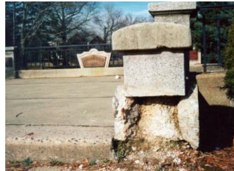
STATE OF DISREPAIR...The Friends of Mindowaskin Park in Westfield has requested that the Town Council include funds in the 1998 Municipal Budget to restore the concrete overlook of the park on the East Broad Street side.
