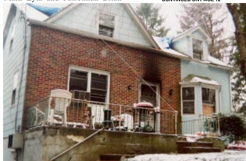
SEVERELY DAMAGED... This two-family home on Raritan Road sustained severe damage following a fire last Thursday. The blaze was reportedly caused by a faulty refrigerator. No injuries were reported.
