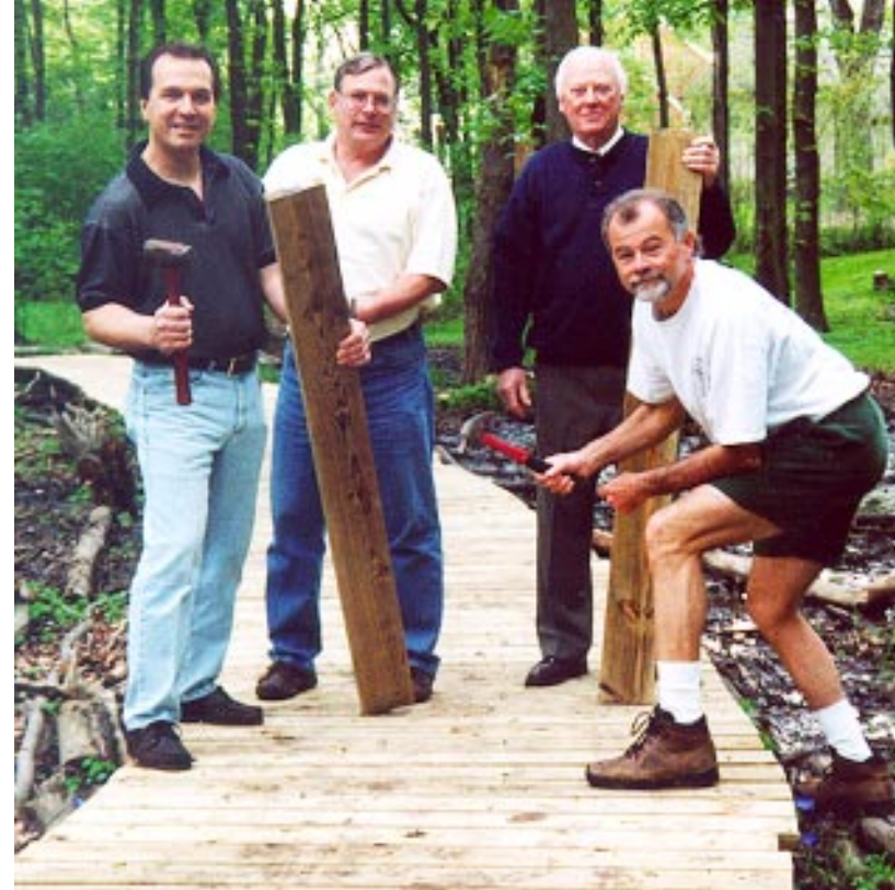
BOARDWALK BUILDERS... Approximately 100 feet of boardwalk was recently constructed over the wettest section of trail at the Fanwood Nature Center on Cray Terrace. The builders, pictured left to right, are: Paul Nadolny, Pete Vanderheyden, a member of the Fanwood Environmental Commission; Bill Kirner and Environmental Commission Chairman and Nature Center Groundskeeper Dean Talcott.
