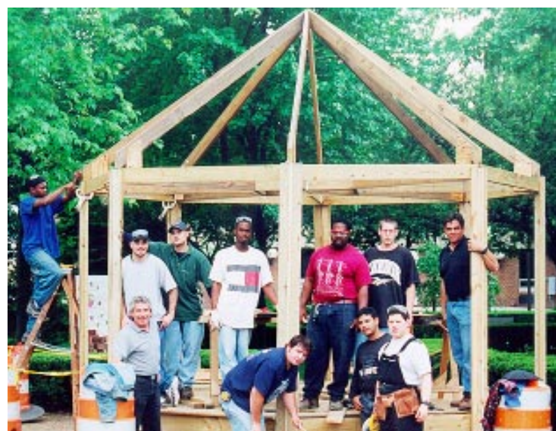
THE HIT PARADE... The Scotch Plains gazebo should be finished just in time for the Memorial Day Parade, if the weather cooperates. Located on the Park Avenue and Front Street corner of the Village Green, council members said they want to use the donated structure as a parade viewing stand. President of the Scotch Plains Business and Professional Association Ray Pardon, says residents can use the gazebo for weddings and photo settings. He also hopes the gazebo will become a landmark for the downtown area. Pictured are students from Union County Vo-Tech who volunteered to build the gazebo.
