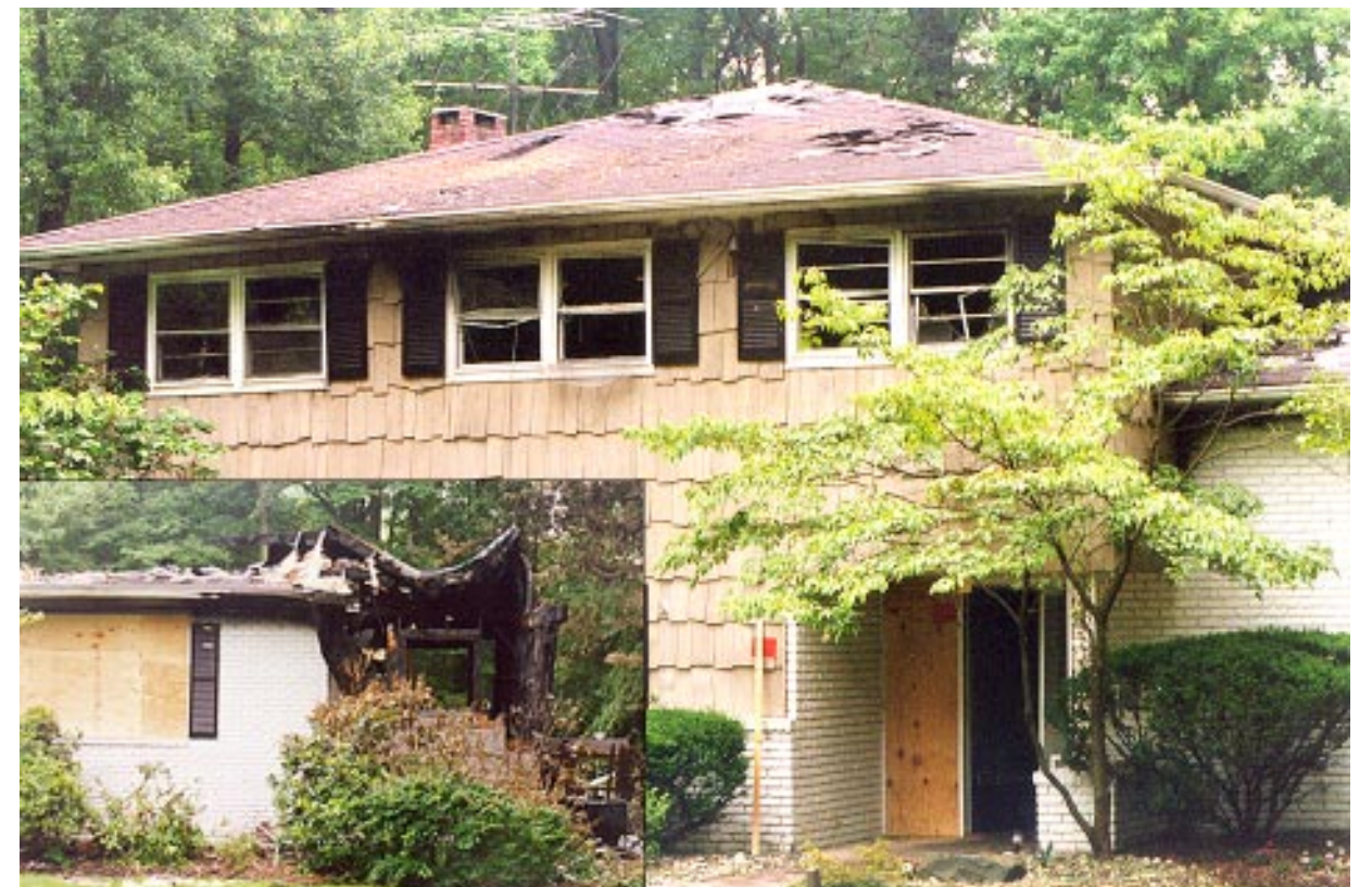
BURNED BY LIGHTNING...This home at 1260 Sleepy Hollow Road in Scotch Plains sustained significant damage after being struck by lightning last Saturday night. A lightning bolt is believed to have struck a tree, bounced over an air conditioning unit before entering the house. The split level home sustained the most damage to the family room, located on the right side of the home, shown in the inset.
