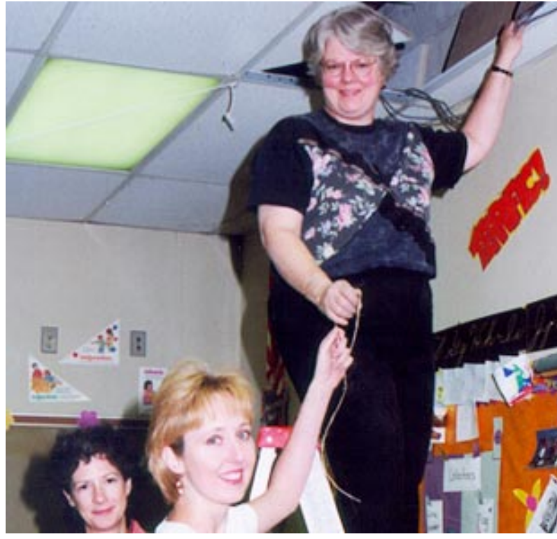
PARENTS HELP WITH NETDAY PROJECT... Earlier this month, parents of students at School One Elementary in Scotch Plains volunteered their time on a Saturday to help wire the school's classrooms for the Internet. Pictured here helping to install the basic wiring, left to right, are: Katherine Balch, Eileen Ayala and Nancy Bauer.
