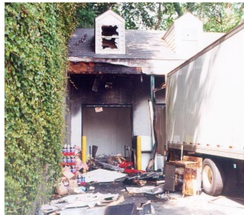
FIRE DAMAGE...The storage room just inside the loading dock at Edwards Super Food Store on Elm Street sustained damage following a fire Tuesday morning.
