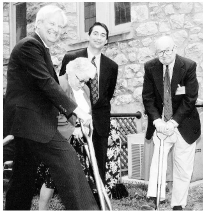
GRAB A SHOVEL...Westfield Mayor Thomas Jardim, standing at center, observes a July groundbreaking for a new entrance and elevator at the First United Methodist Church of Westfield on East Broad Street. Also pictured, left to right, are: Reverend David Harwood, Senior Minister, Dot Reeder, Financial Secretary of the Access-Now Building Committee, the Mayor, and Doug Merrill, Chairman of the Access-Now Building Committee. The ceremony was followed by an old-fashioned ice cream social. The morning events were organized by a committee chaired by church member Carolyn Greasham.
