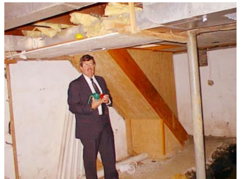
STILL NO SATISFACTION... Westfield resident Burton Michaels stands in the basement of his Everson Place house three years after a heating oil tank burst when it was apparently overfilled during a routine delivery of oil. A hole in the ground filled with water, sewage and traces of oil sit where the former finished TV room existed.
