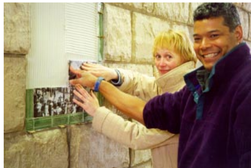
RECREATING HISTORY... Stacey Farley, a native of Westfield, and Dale Wong of Ceramic Tile Design, Inc., install one of 18 tile murals in the renovated Westfield Train Station last spring. Ms. Farley, who created the murals depicting moments in Westfield's history from 1864 to the 1920s, will discuss the project at the Tuesday, October 6, meeting of the College Woman's Club of Westfield, to be held at 8 p.m. in the Community Room of the Westfield Municipal Building.
