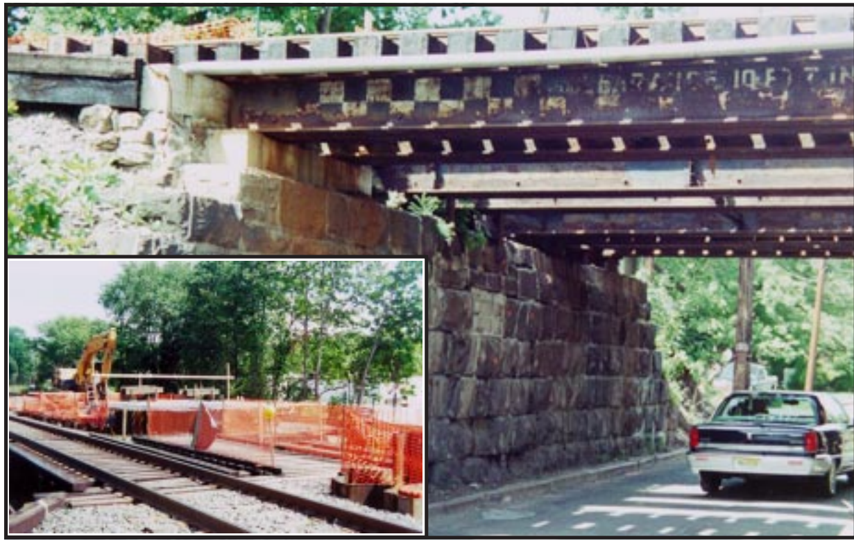
ON TRACK WITH REPAIRS...The NJ Transit steel girder railroad bridge that runs above Crossway Place near Westfield's Public Works Building is undergoing a $1.4 million renovation.
