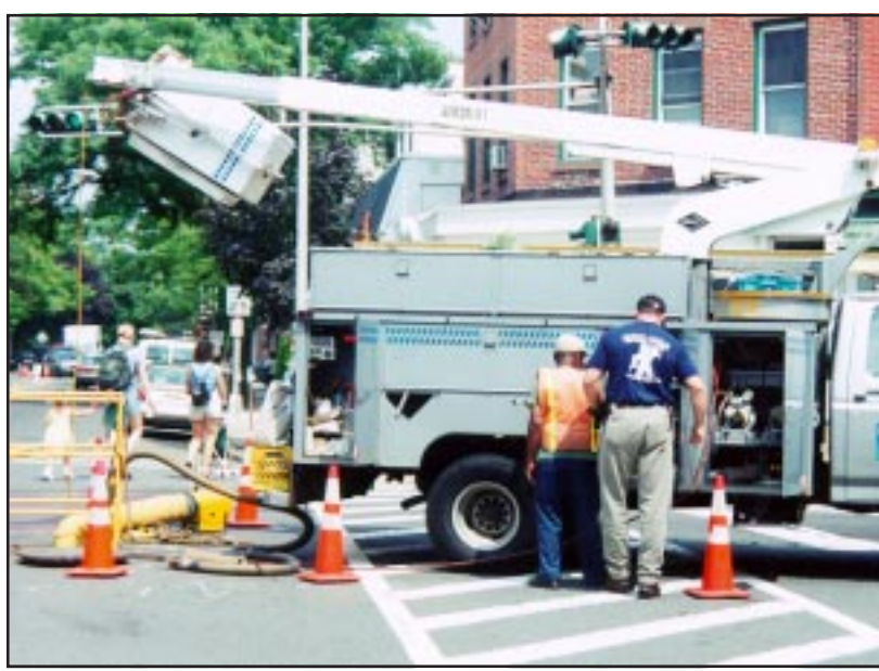
David B. Corbin for The Westfield Leader and The Times UNDERGROUND REPAIRS... The on-again, off-again work that continues to take place below the road surface at the corner of Elm and East Broad Streets in downtown Westfield since late spring will continue for the next four weeks. Bell Atlantic is repairing a large cable and the time-consuming job has been hindered by tight space and, on two occasions, leaking sewer water.
