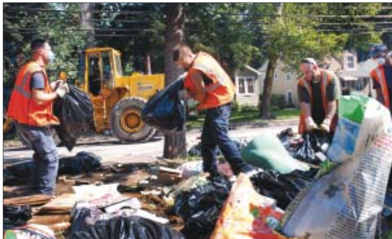
PITCHING IN...County workers remove debris from in front of homes along Springfield Avenue in Cranford. Dozens of trucks and front-end loaders assisted Cranford, which had hundreds of homes and businesses damaged during severe flooding.
