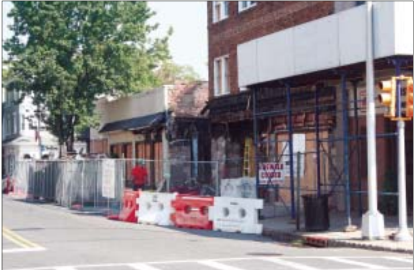
STARTING OVER... Ferraro's Restaurant in Westfield began demolition this week of its building that was destroyed in a fire that occurred in May.
