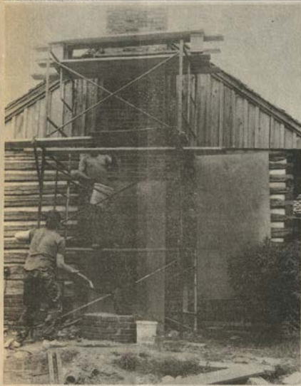
CHIMNEY WORK: The Trigg County Tourist Center in Cadiz received much-needed chimney renovation this week. The decaying chimney was taken apart brick by brick and put back together using the original bricks, repairing the century-year-old building.
