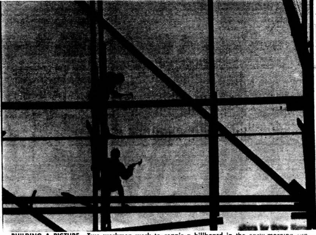
BUILDING A PICTURE —Two workmen work to repair a billboard in the early-morning sun. Caught at the right angle, it appears as though the men themselves are part of an abstractist painting. However, we have been assured that the men are, indeed, quite human and that the billboard is once again spreading its commercial message.
